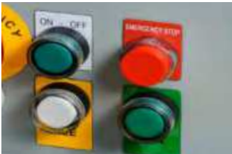
Control panel labels
