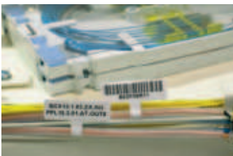
Fibre optic cable markers
